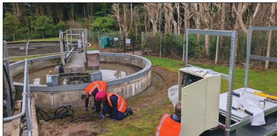
Hutton team working on a control unit - Photo James Hutton Institute
