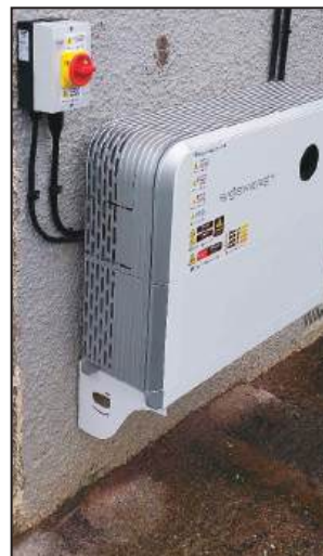
Battery storage for the extra power generated by the solar panels makes sound economic sense
