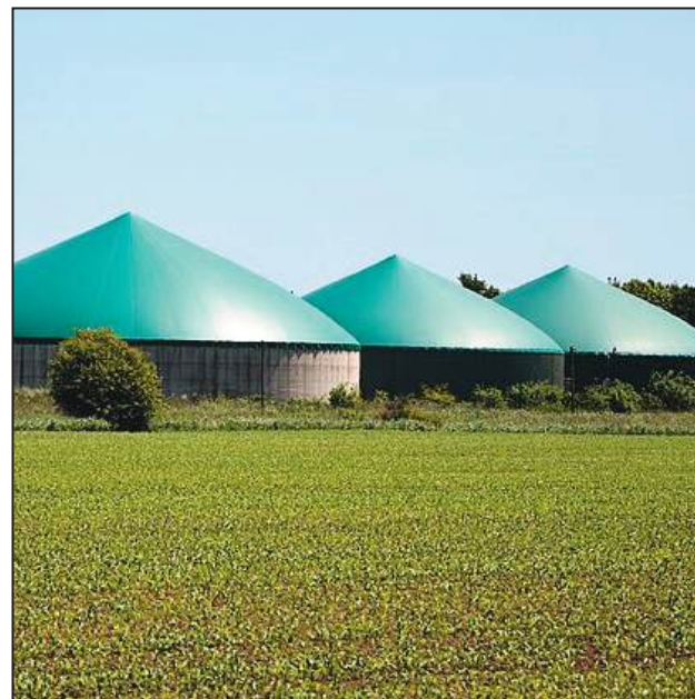
An example of a biogas installation
