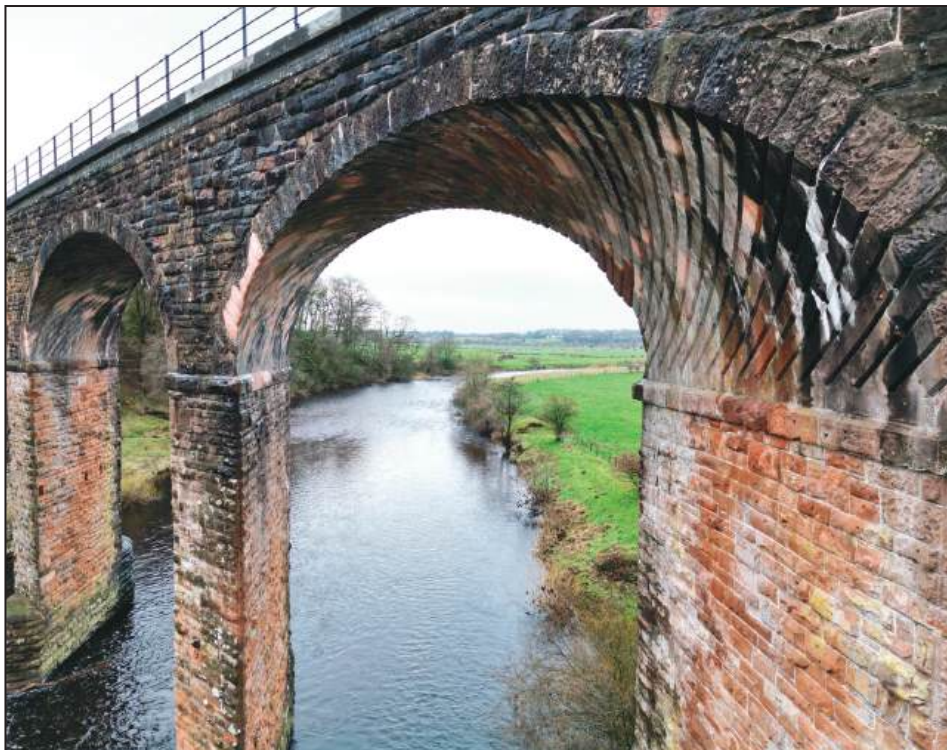
The iconic Riddings viaduct has been restored for future generations to enjoy
