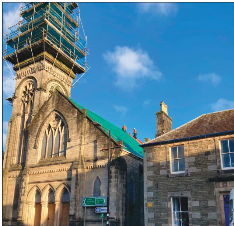
The unsafe state of Langholm's Erskine Church does not come under Environmental Health's remit
