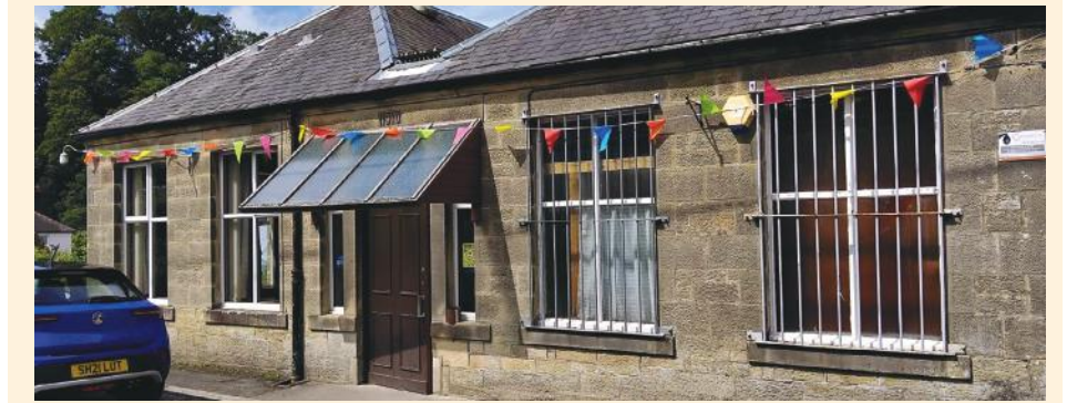
Langholm Social Club is raising funds to repair part of the roof of their building. They're looking for community support as they offer space for lots of other community organisations to fundraise and hold events. Some of the groups that use it include the carpet bowling club, the fiddle and accordion club, the town band, the pipe band and the Castle Craigs club. Fiona Patterson has started a gofundme page to 'raise the roof'. At the time of going to press £100 had been raised out of a target of £3000. If you'd like to donate, go to https://gofundme.com/f/5nweey-raise-the-roof
