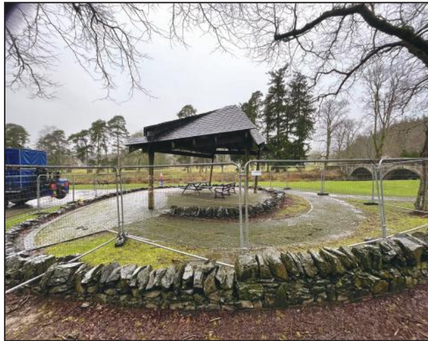
A-BAND-ONED: The bandstand on the Kilgreen needs to be demolished or repaired before November 5th - Photo: D. McVittie
