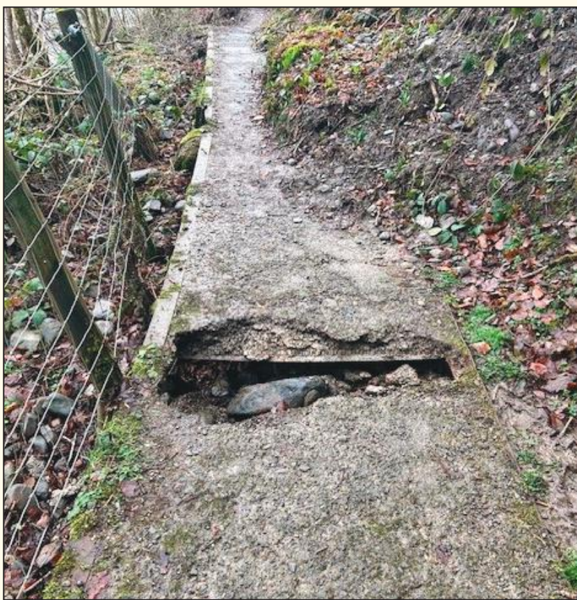
SERIOUS: The concrete walkway above the Esk has become unsafe for walkers Photo by Gavin Graham
