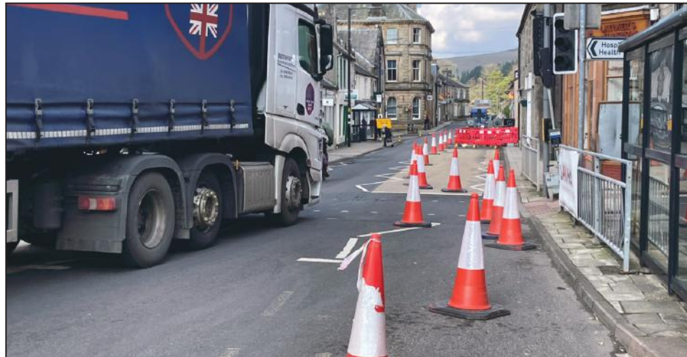
POINT IN QUESTION: The current roadworks on Langholm High Street won't be helping D&G's carbon footprint
