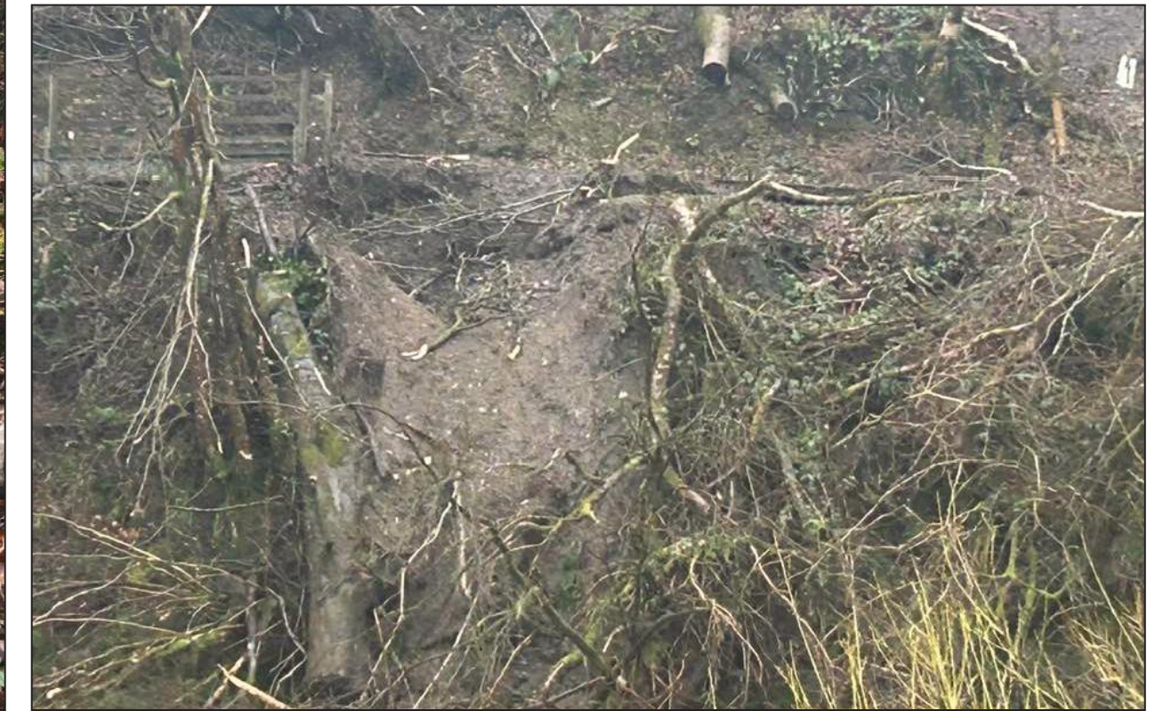
EASTON'S WALK: Taken from the opposite bank of the Esk. You can see the full extent of the slip
