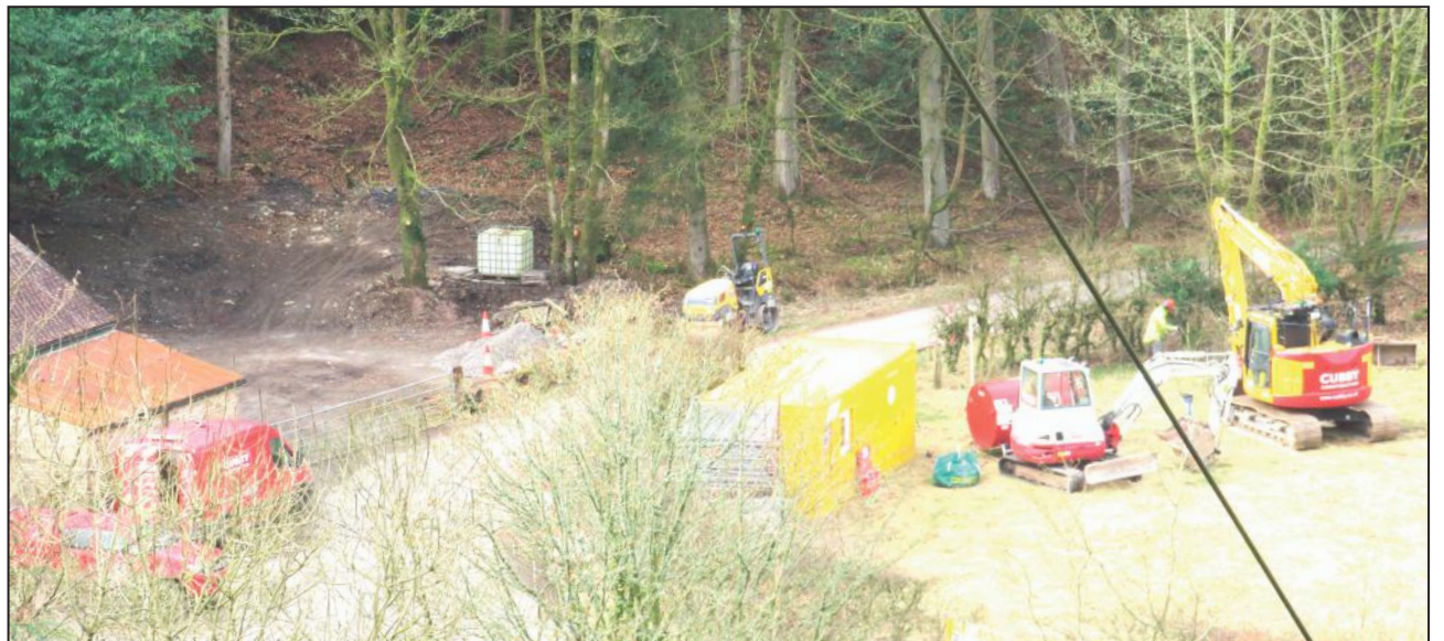
DIG IT: The arrival of heavy machinery at Murtholm is a welcome sight, although traffic disruption is also predicted for the next six months
