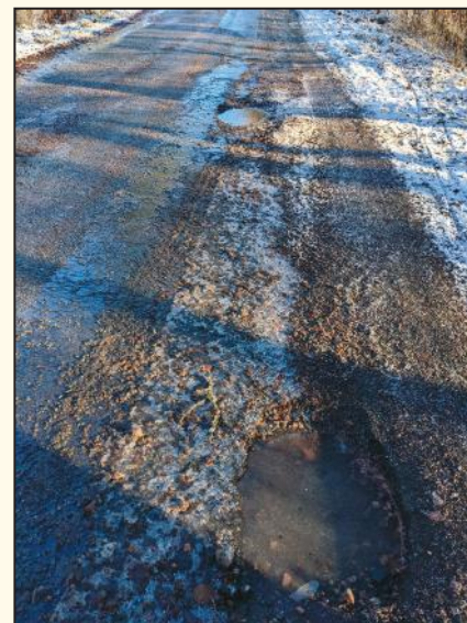
CRATER: This foot-long pothole is just one of the many blighting the B6357 road at Gilnockie
